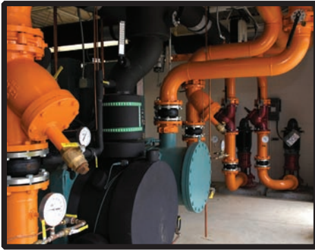
Inside the new Chiller Building.
