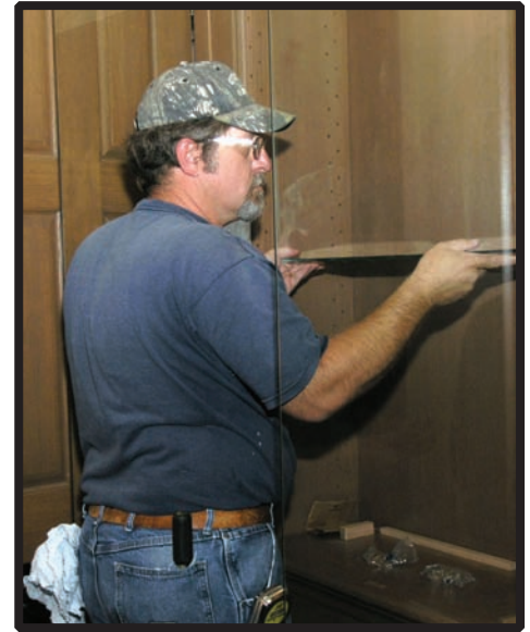
Scott Davis of the Carpentry Shop installing cabinet shelves as part of the technology upgrade to Franklin 106.
