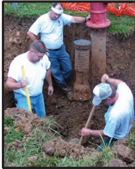
Frank Ducharme, Mike Franklin, and Mike Self of Utilities Division repairing a firehydrant.
