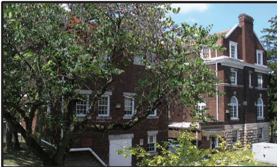
The eastern side of 1022 East Third Street will have the windows reglazed and painted in addition to tuckpointing.
