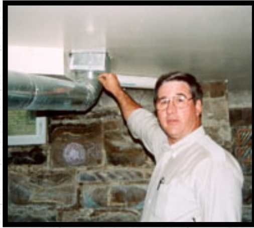
Dale Lisby, Assistant Manager of Building Maintenance, directs our attention to some of Knee High's new ductwork.
